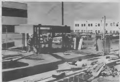
The new gate house at Gate 3 in front of the General Office Building is in center of road.
